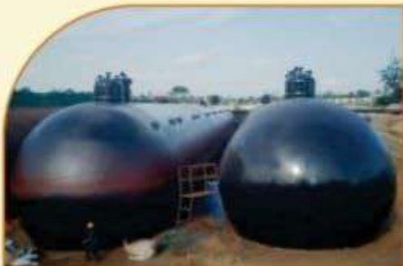
Mounded Storage Tanks
